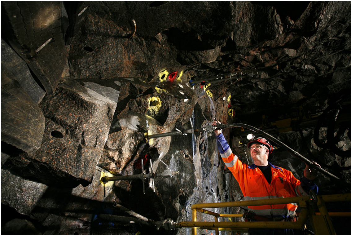
Figure 4-1. Checking of the equipment at the tunnel front in the experiment Sealing of Tunnel at Great Depth).
